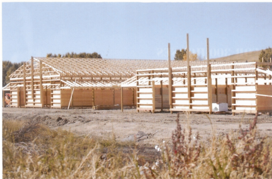
Anderson Ranch is under construction. Two of their four new barns are shown here.
